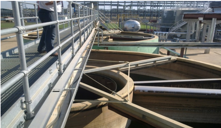
Discharge flotation unit
